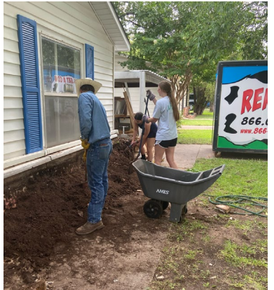
Caleb, Holly, and Sydney help renovate a house that will be used to support missionaries.
